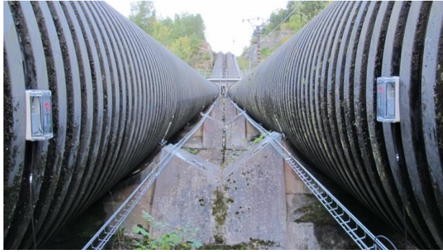
Picture 4: Cable path, and 2 boxes including sensor and pre-amplifier
